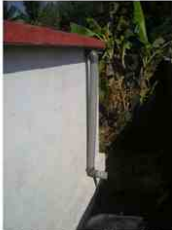
Fig 13: Overflow pipe with mesh
