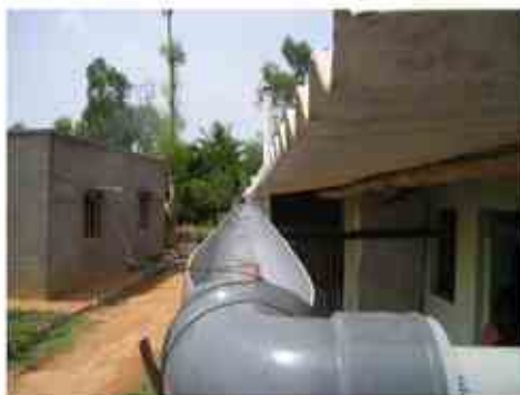
Fig 6: A clean PVC gutter to catch every drop of rain
