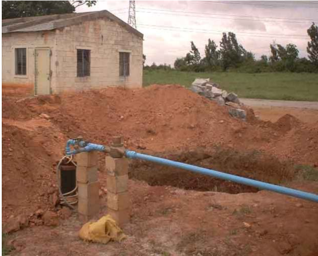
Borewell and recharge pit
