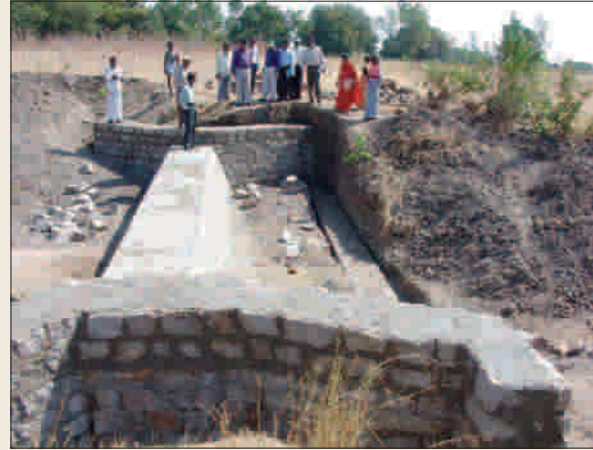
Check dam in Chowderpalli
